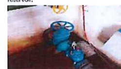
Damaged PRV Valve, which causes overflow of water
